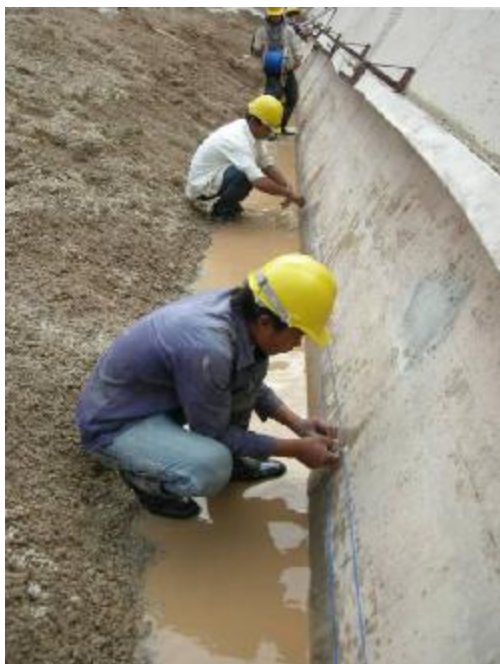
Figure 6. Men at work at dam's plinth to install the blue distributed sensing cables
